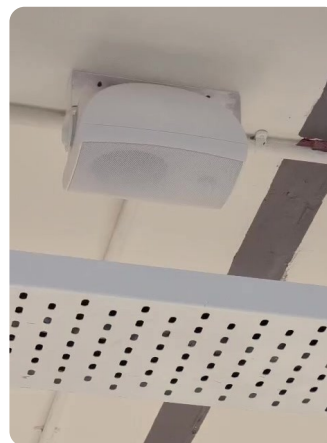
Ceiling-mounted PA speaker on the shop floor
